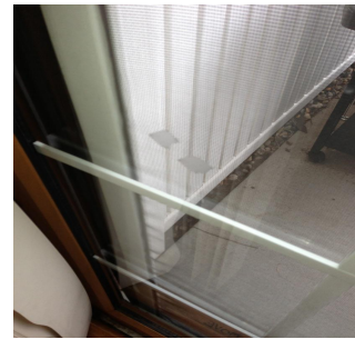
Tape on Windows/Glass
