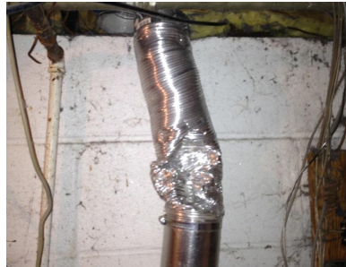
Dryer Venting Not to Code
