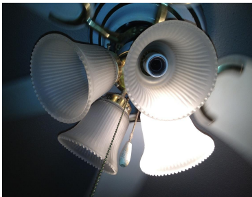
Missing/Burned Out Light Bulbs
