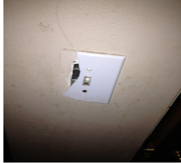
Cracked Switch Plates
