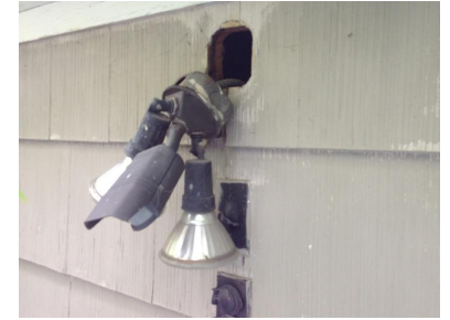
Broken Exterior Light Fixtures
