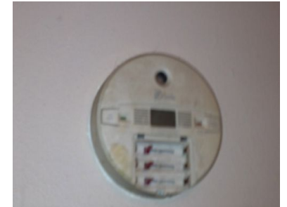
Batteries Missing from Smoke Detector
