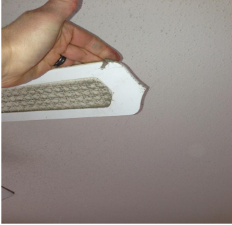
Dirty Ceiling Fans
